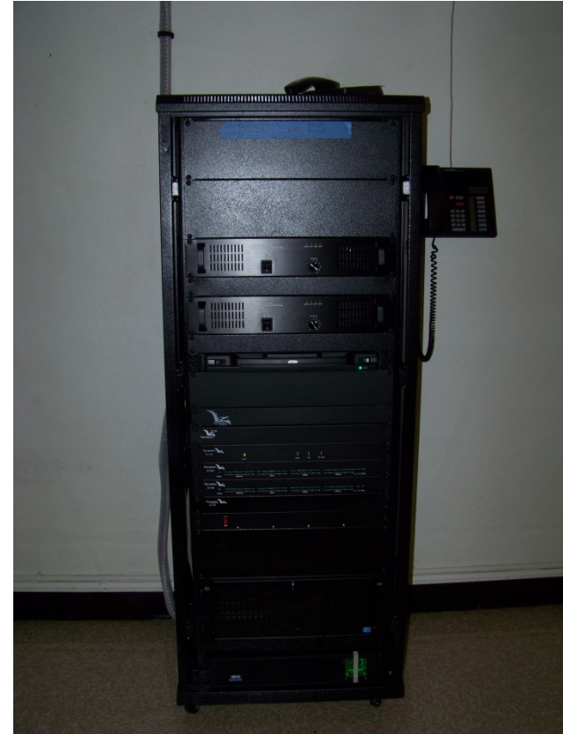
Intercom Head End Equipment w/ Paging Phone adjacent – Lee E.S.
